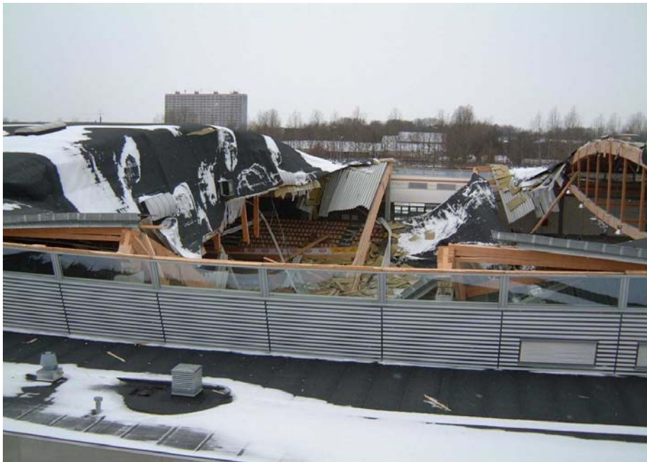
Figure 1. The roof of Siemens Arena after the collapse of two trusses. An intact truss is seen to the right.
