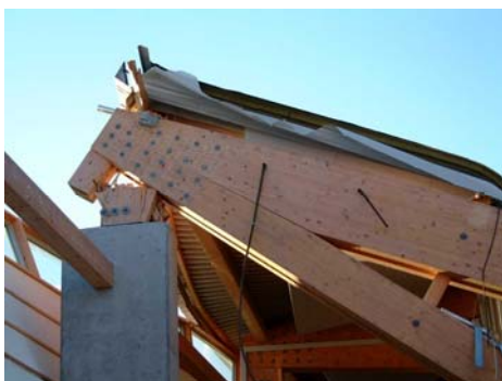
Figure 2. The corner where concealed steel plates connects the timber parts. Between the visible bolts numerous dowels are placed.
